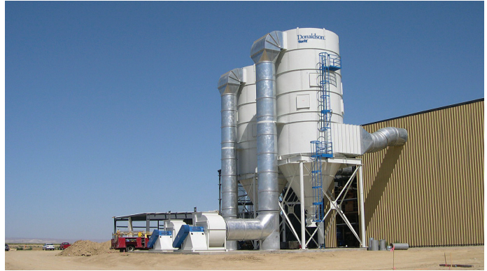
882LP12 at Almond Plant 140,000 cfm/each (237,811 m 3 /h each)
