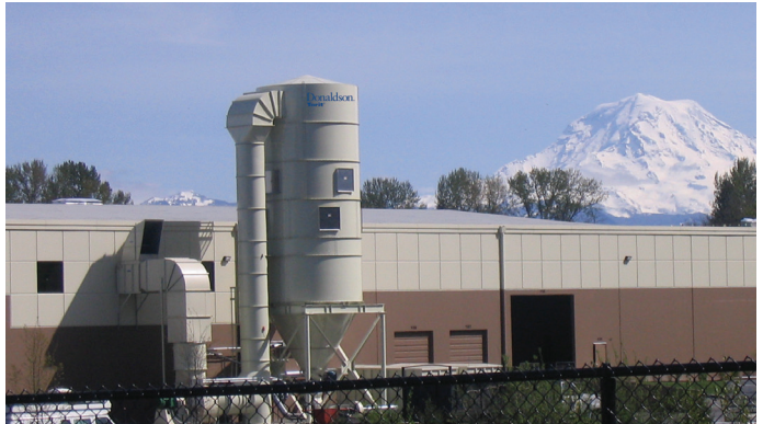
528LP12 at Cabinet Factory 70,000 cfm (118,906 m 3 /h)
